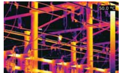
Substation Thermal Image
