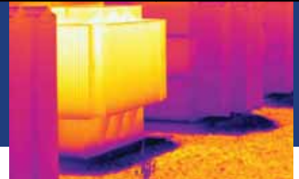
Transformer Thermal Image
