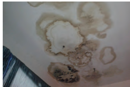
Pic. 1 : Mold development on the ceiling...
