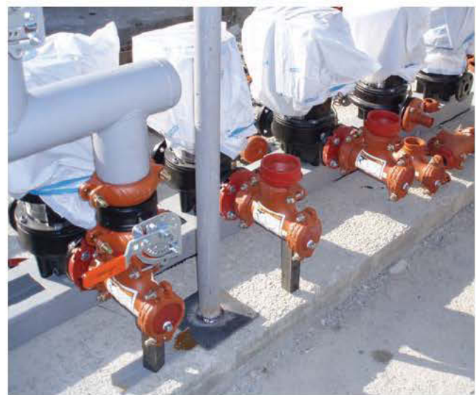
The flame free assembly of the Victaulic grooved mechanical system allowed patient care to carry on unhampered during installation...
