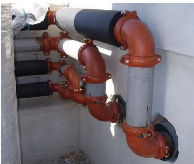
The flame free assembly of the Victaulic grooved mechanical system allowed patient care to carry on unhampered during installation...
