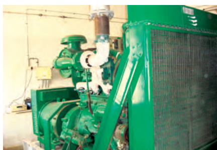
DG radiator heating the surroundings inside...
