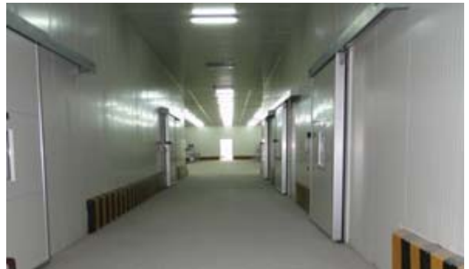
State-of-the-art pack-house, cold store and ripening facility at fruit and vegetable market, Ludhiana
