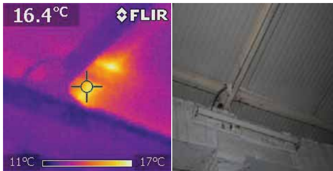
Small insulation leakages can easily be detected before they escalate into something worse.
