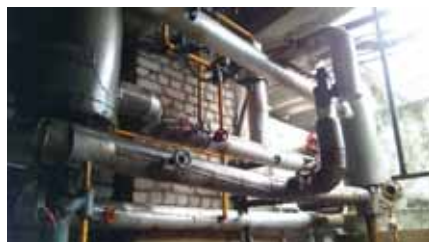
Plant piping before modification
