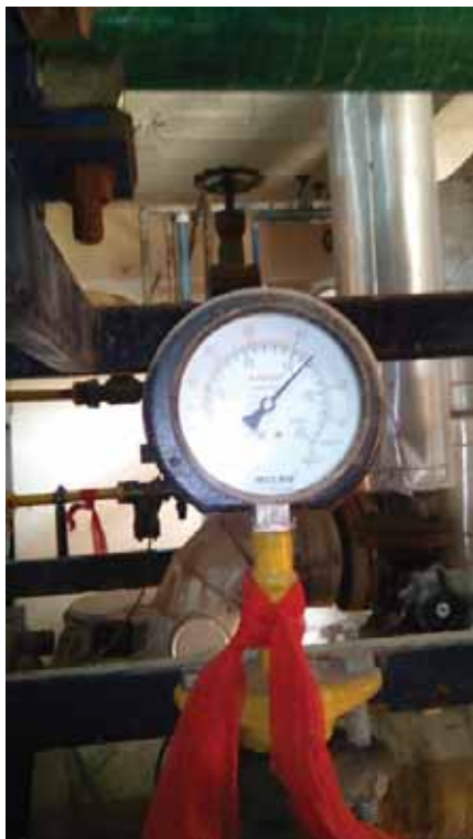
Plant discharge pressure before plant modification
