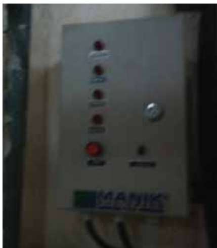
Cold room Safety Alarm system
