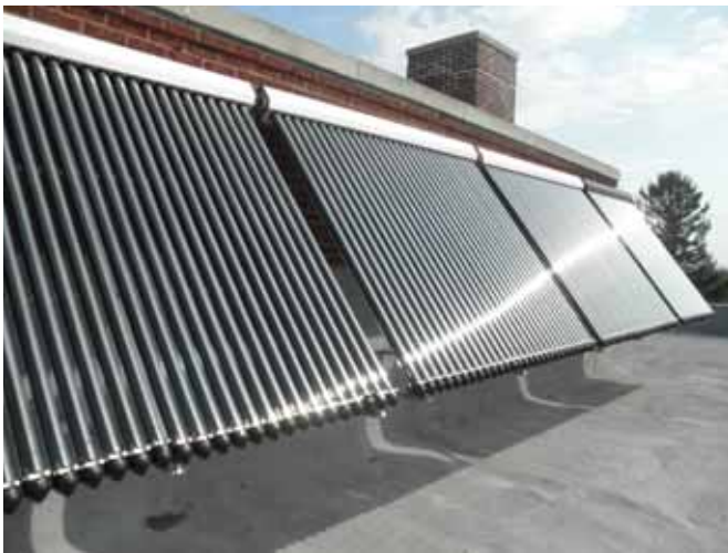
Wall-mounted evacuated tube solar thermal system
