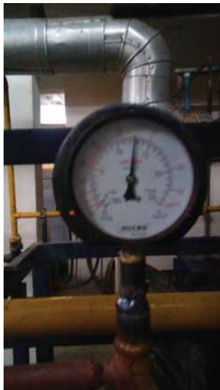
Plant discharge pressure after plant modification
