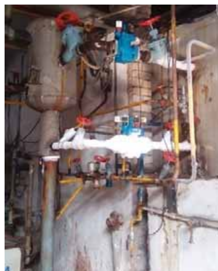
Plant piping after modification
