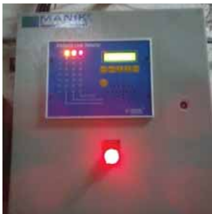
Ammonia Leak detection system
