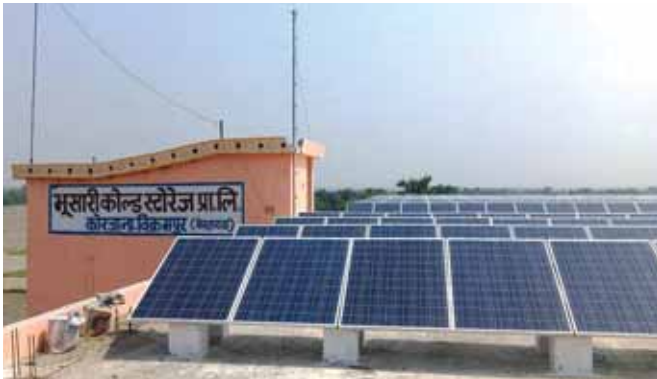
The 100 kWp grid-connected rooftop solar system at Bhusari Cold Storage generates approximately 147,000 units (kWh) annually. Savings in power bill during the first year are expected to be approximately INR 11 lacs and INR 465 lacs over the project lifetime (25 years)...
