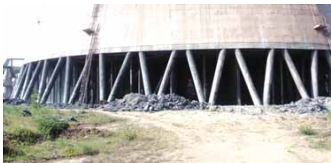
Figure 7: View of air induction area of a natural draft cooling tower...
