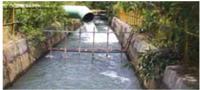
Figure 10: View of a canal water cooling system...
