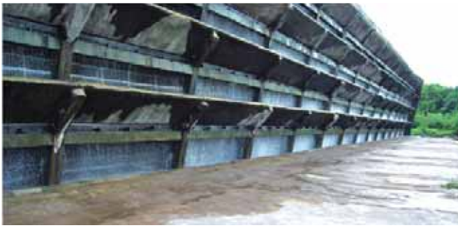
Figure 9: View of air induction area of a forced draft cooling tower...
