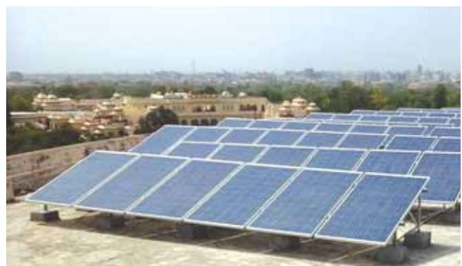
100 kWp Grid-Connected Rooftop Solar System (Front View)...
