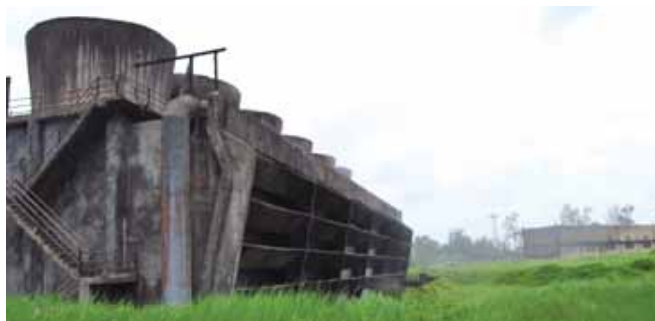
Figure 8: View of a forced draft cooling tower...
