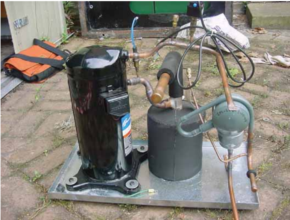
A photograph showing the connection of DX GSHP installed at the School of Built Environment...
