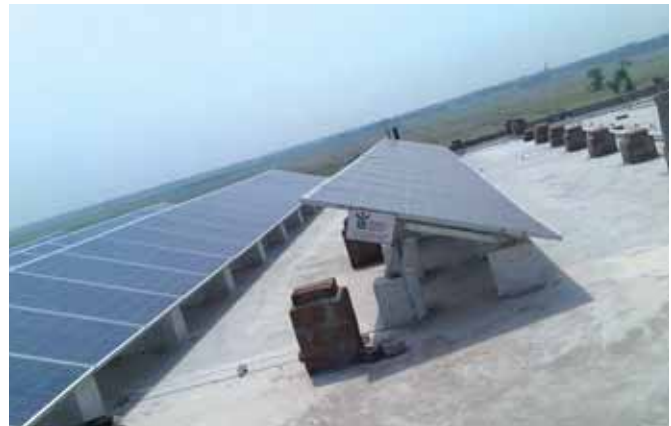
100 kWp Grid-Connected Rooftop Solar System...
