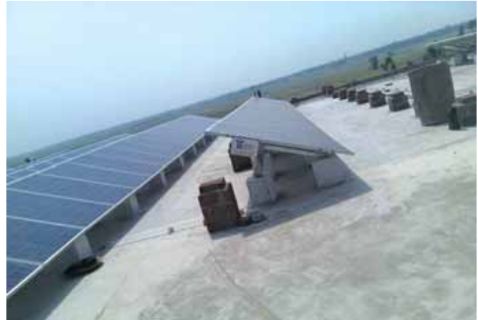
100 kWp Grid-Connected Rooftop Solar System (Side View)...
