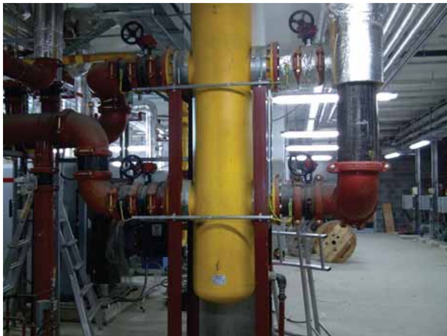
Avoiding pipe flaking and descaling caused by welding means cleaner water runs through the hospital's piping systems...
