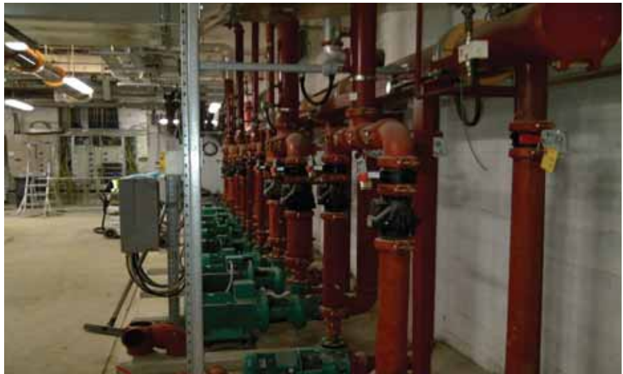
Victaulic check valves, butterfly valves and strainers were used in the hospital's plant room...
