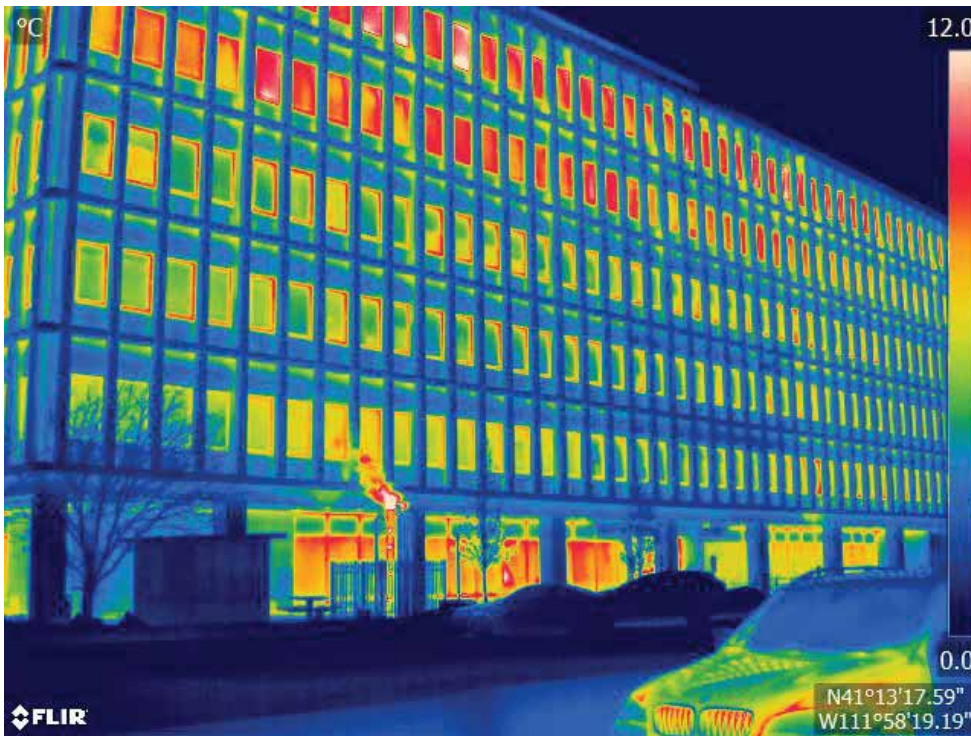
A thermal image of the Hansen Federal Building in Ogden, Utah, where Berkeley Lab performed a window retrofit study... (Credit: Berkeley Lab Windows and Envelope Materials Group)
