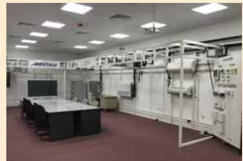
Training centre for multi air-conditioning system for buildings in the FG (ME) office...
