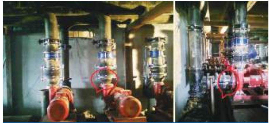
Fig. 8: Reducers/Enlargers at Pump Suction & Discharge
