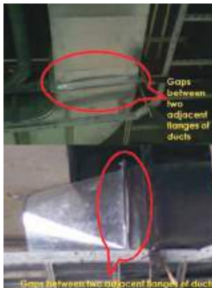
Fig. 6: Gap Between Two Flanges of Ducts Where Air Leakage Occurs
