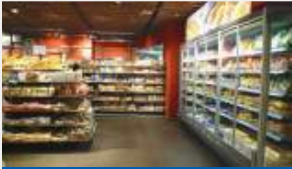
Fig. 3: CO 2 systems and chilling cabinets with glass doors help Migros save a lot of energy.
