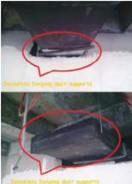
Fig. 4A: Senseless Hanging Duct Supports
