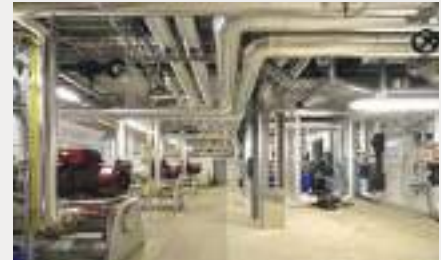
Fig. 2: The new ammonia plant at Fleischrocknerei Churwalden combines refrigeration and the use of waste heat.
