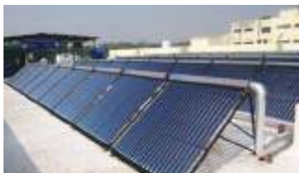
Fig. 2: Solar thermal field
