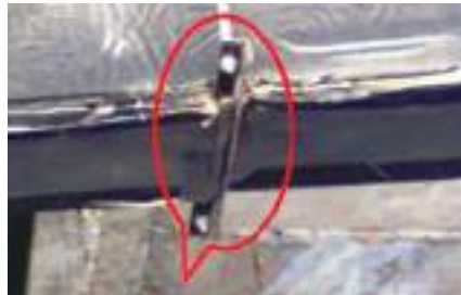
Fig. 5: Partly Insulated Metal Support in Contact with Cold Air Duct
