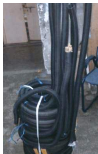
Fig. 11: Polypropylene pipes coiled and stacked above one another
