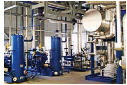
Fig. 4: Inside the machinery room of ASDA's Lutterworth Distribution Centre... Source: Star Refrigeration (2007)
