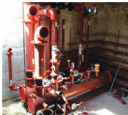
The mechanical room was designed to fit into a very small space...
