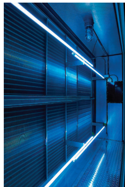
Fig. 2: Example of the 'blue hue' of a UV-C lamp installation. The intensity of the blue does not indicate the efficacy of the light. Modeling is the most accurate and efficient method to determine UV-C energy levels... Courtesy: UV Resources
