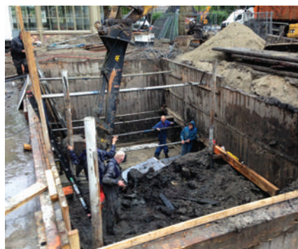
A new basement area had to be created to house the mechanical room...
